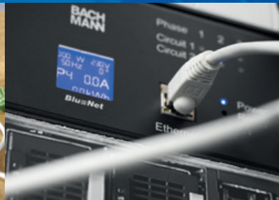
IT POWER SOLUTIONS
